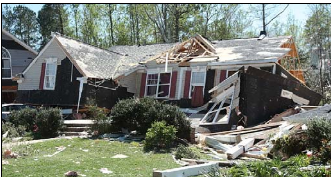
Engine 25 was dispatched to Pritchard Court for a building collapse. Finding only moderate damage, they were directed to the next street, Serendipity Drive. They found many damaged homes, including this one, photographed the next day. Two dogs were reported missing. The crew carefully searched the debris, and found both of the dogs, though only one had survived.
